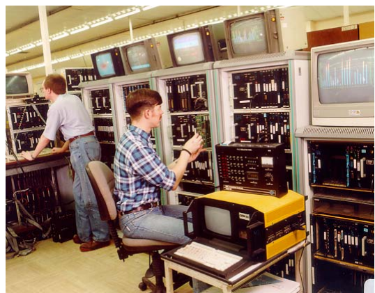
GEM80 Systems Test Area
